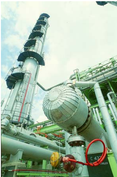
Figure 1: Ammonia column (Courtesy of Emerson Process Management)
