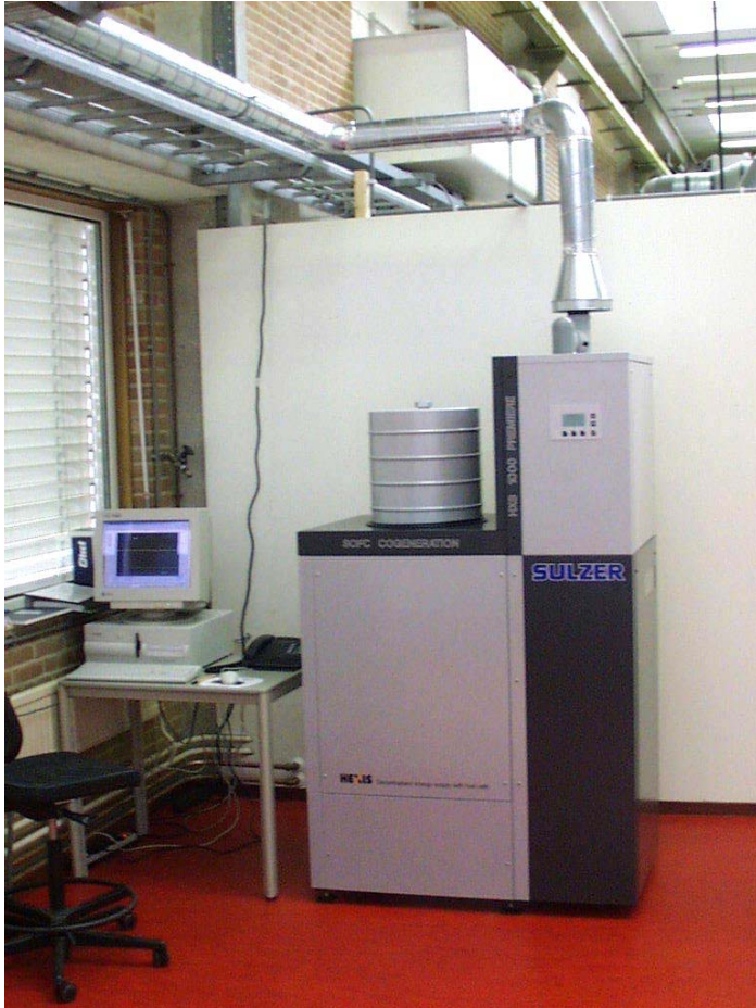
Figure 13 Sulzer HXS 1000 Premiere system at ECN, NL.
