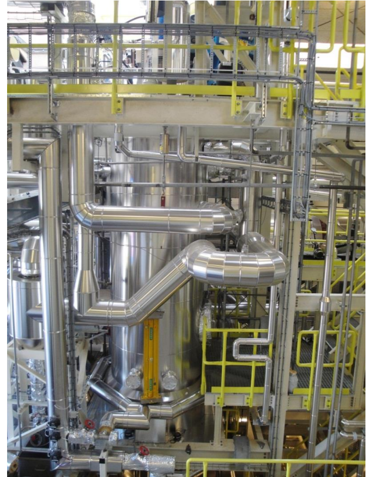
Torrefaction section of the demo plant
