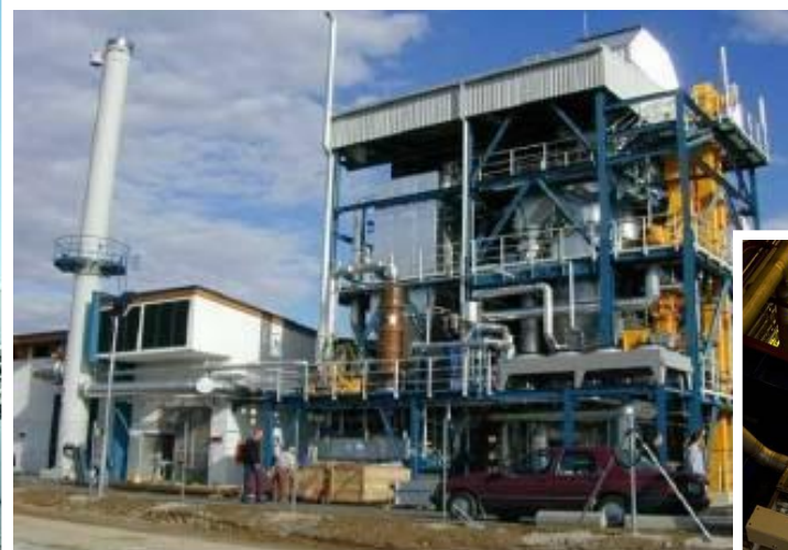
Repotec FICFB gasifier, Güssing (Austria), 2 MW e
