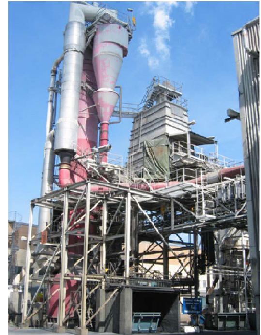
CFB Metso, Varo (Swe), co-firing lime kiln 35 MW th_biomass
