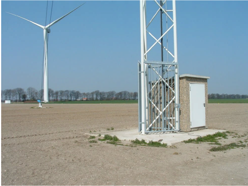
Figure 4-3 Measurement cabin on the meteorological mast 1 foundation. The signal reception and front-end of the DANTE data-acquisition system are inside. On top the precipitation sensor is located.
