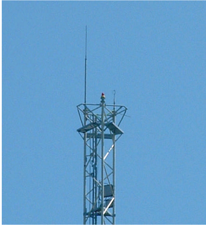
Figure 4-1 Top of the meteorological mast 1 with 3D sonic sensor, aviation warning light and lightning conductor. The boxes lower in the mast contain the signal connection and high voltage protection.
