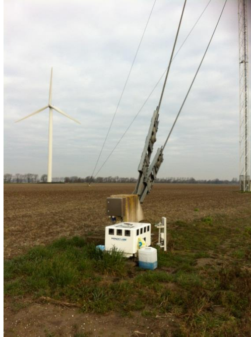
Figure 16: Windcube V1 LiDAR near the base of the 180deg guy-wire of MM3
