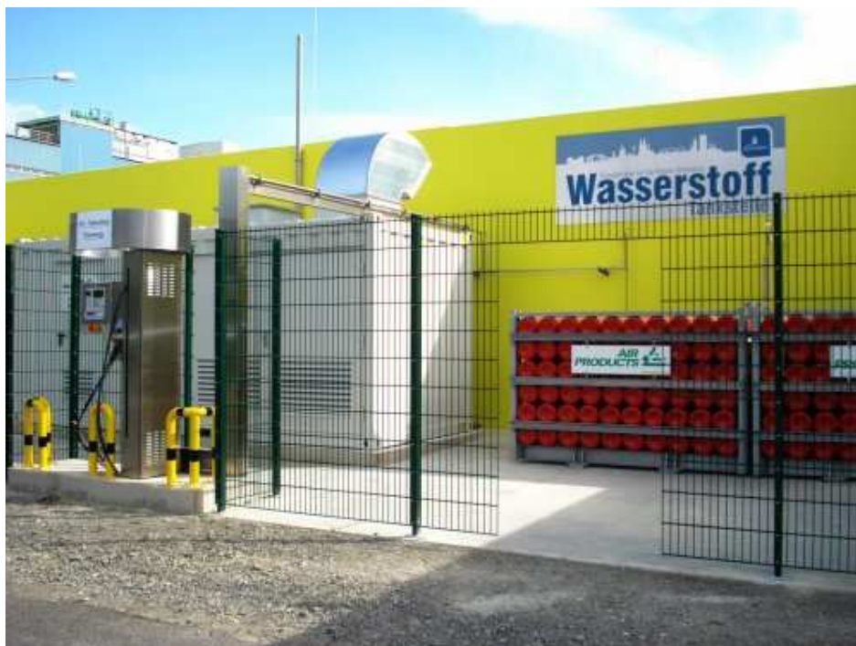
Figure 4.3 Hydrogen refuelling station in Hürth
