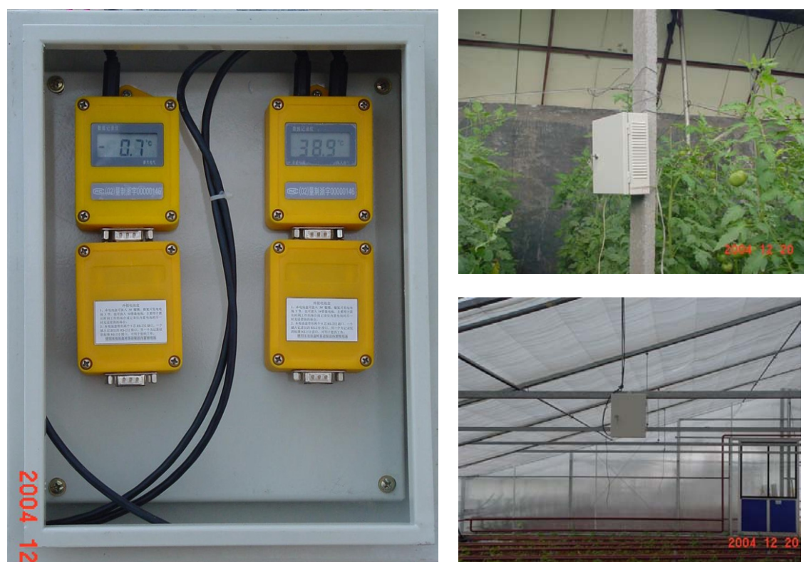
Figure C.1 Left: two data recorders; right: two times the protection box in which the data recorders are placed
