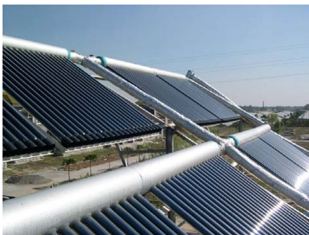
Figure 3.10 Picture of the solar collectors at the roof of Greenhouse II
