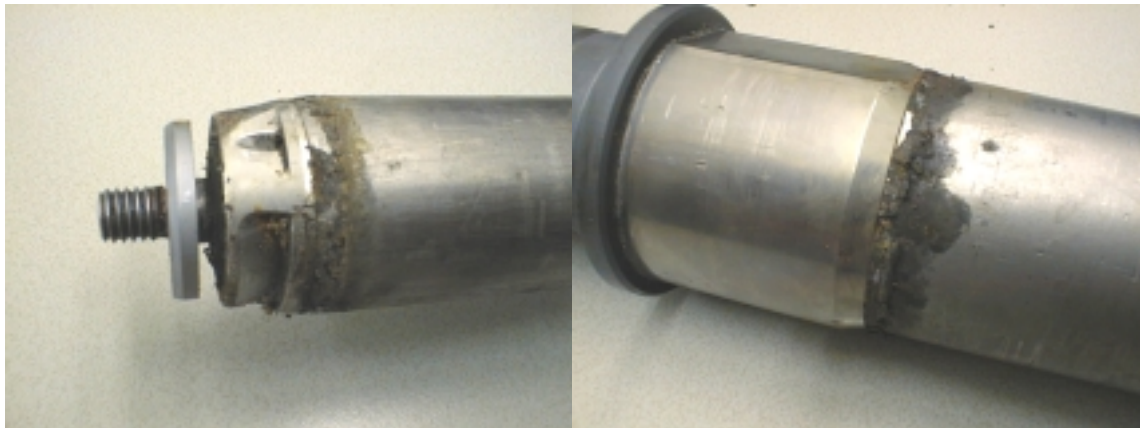
Figure 2.2 Details of the corroded 17.4PH parts
