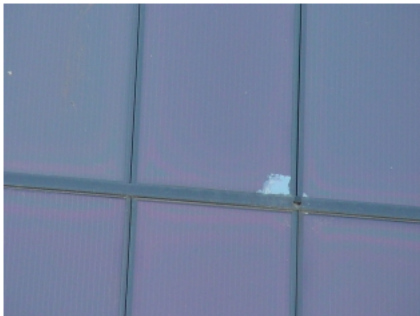
Figure 18: Delamination of a module on the North façade.
