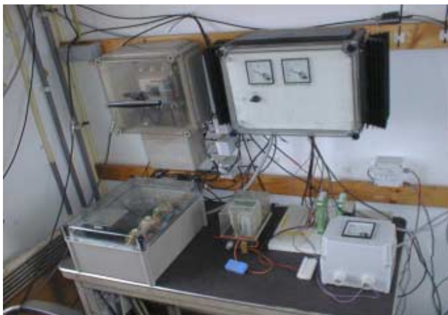
Figure A.3 Turbine switch, rectifier control box and measurement transducers
