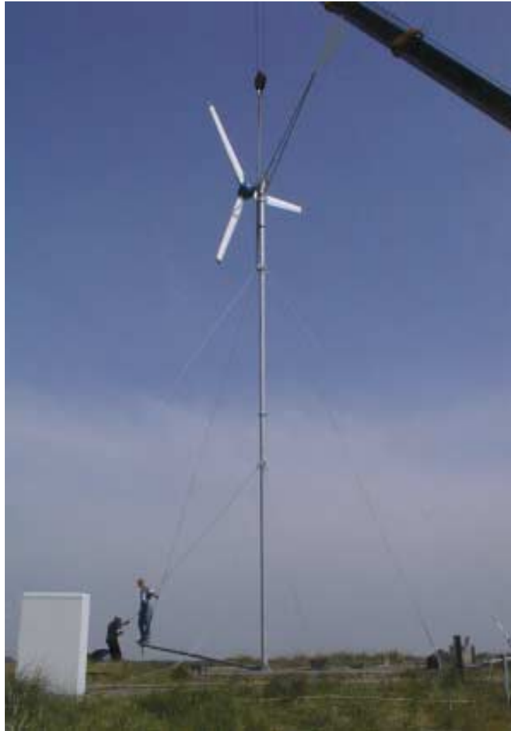
Figure A.1 Fortis turbine installed at ECN testsite
