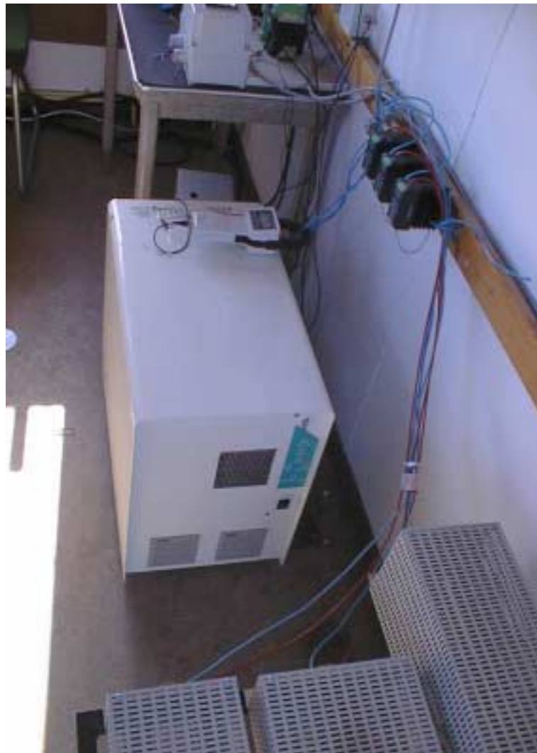
Figure A.5 Sunpower PV UP 5000 Inverter
