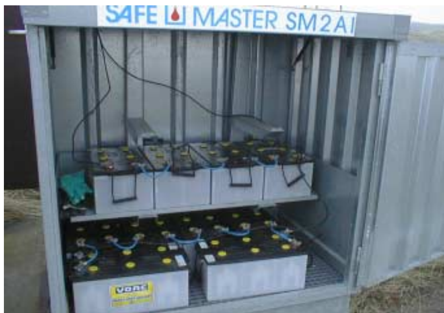
Figure A.7 Batteries
